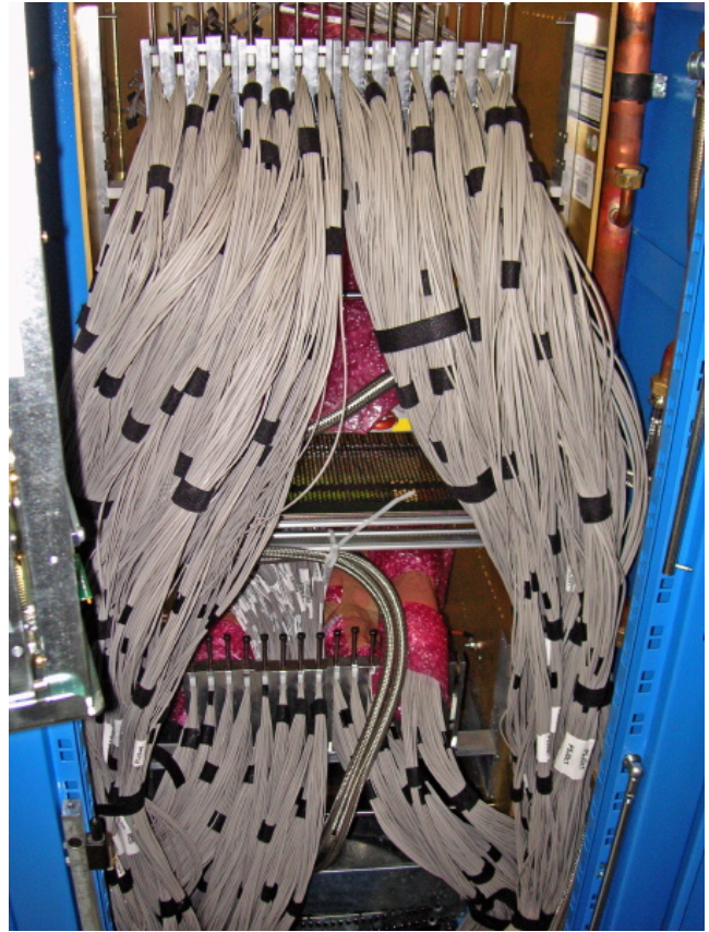
Fig. 5. Full LVDS input cabling at the back of a JEP crate
