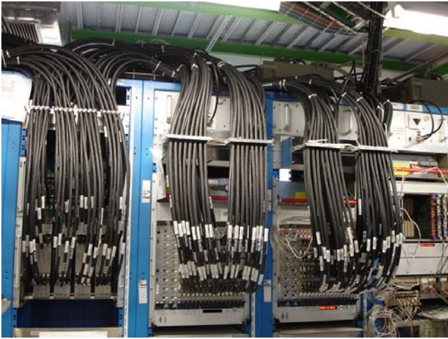
Fig. 4. One quarter of the analogue cable inputs into the preprocessor system. Supporting stocks are located at about 2/3 of cable height
