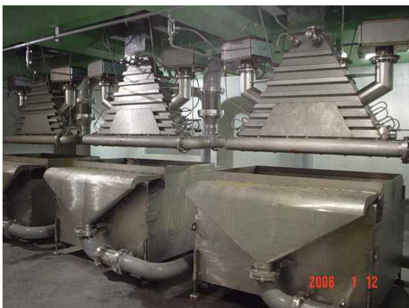
Commercial waste water treatment plant
